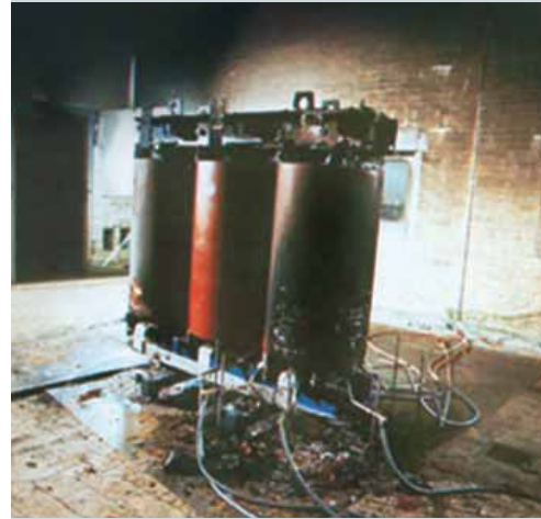
Figure 8: Condition of the test object after the fire behavior test: The overall view of the HV windings also shows that the fires at the outer legs did not spread to the center leg in substantial degree.
